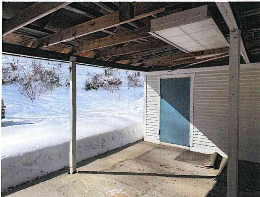
Beam with observable deflections and column settling away from slab
