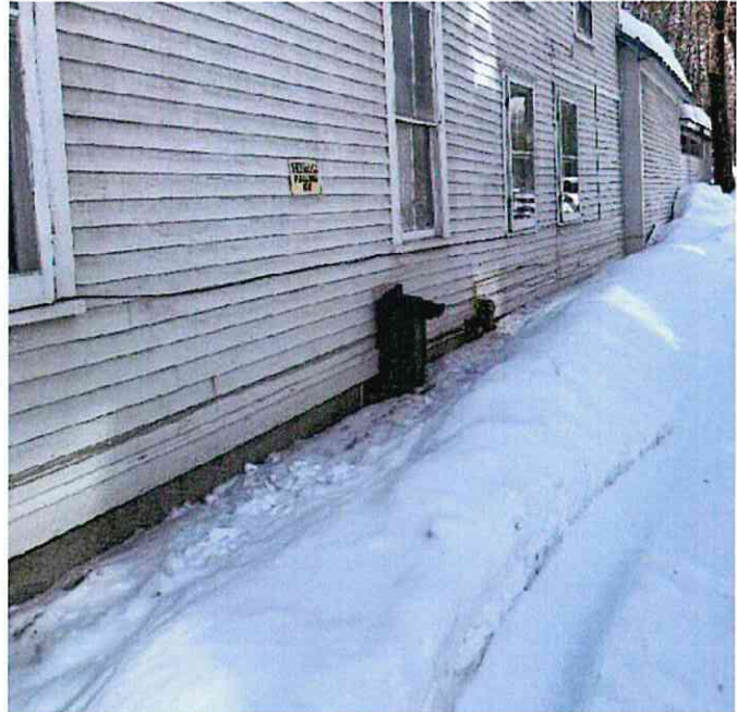
Negative drainage example on east side
