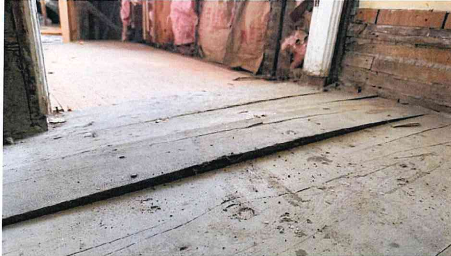
First floor of addition having localized deflections due to foundations below lifting through floor framing
