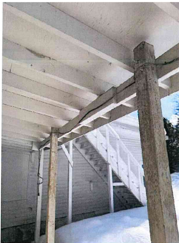
Entry roof rafters bearing on a single ply (improperly spliced) beam, columns bolted, not bearing
