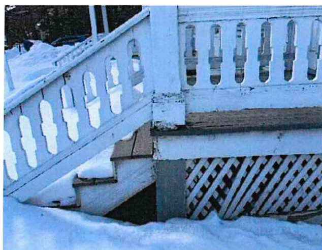
Eastern porch at original building settling at foundations
