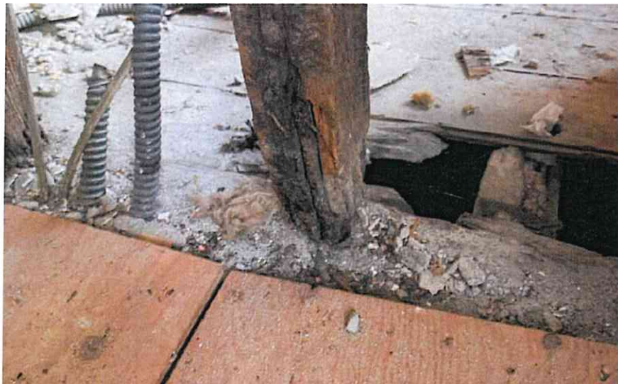
Example of column in addition experiencing significant section loss due to rot/deterioration
