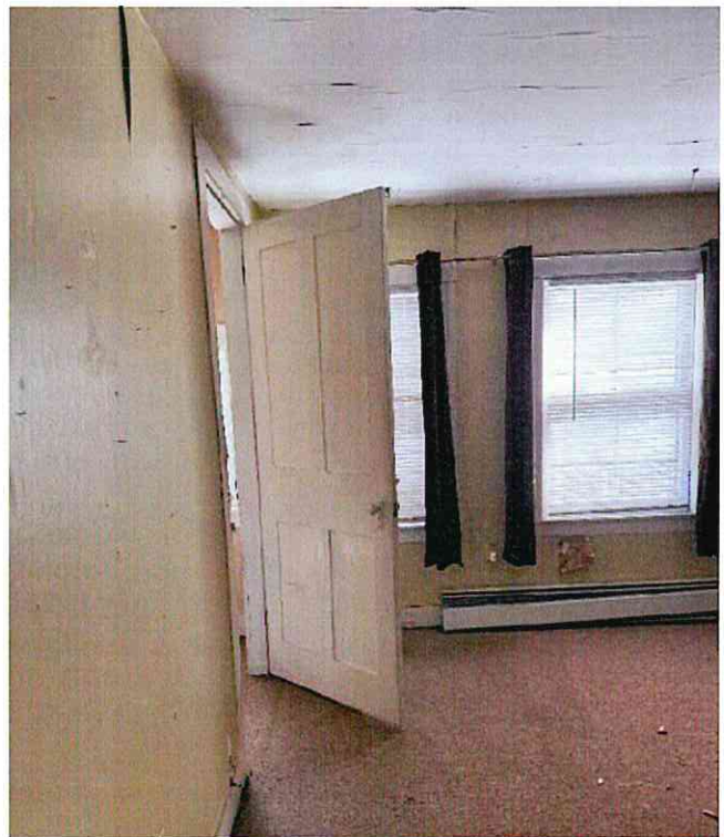
Third floor settling toward interior wall, interior finishes suggest long term high humidity
