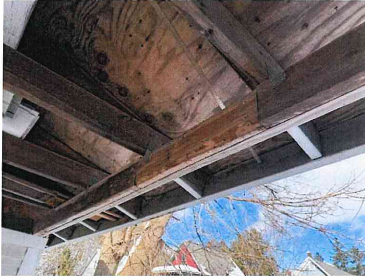
Improper beam ply splice at carport
