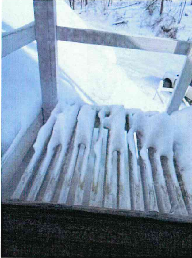
Top landing of fire escape stair with rot and unconventional dense framing without decking
