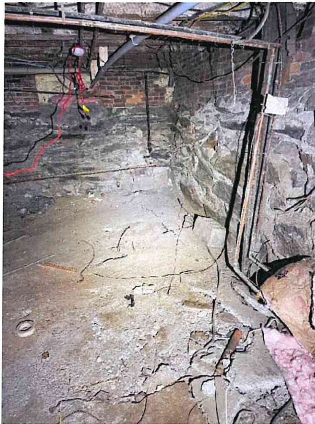
A corner of the original basement with frost activity moving the slab and walls
