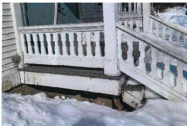
Stair at church hall porch dropping away from porch
