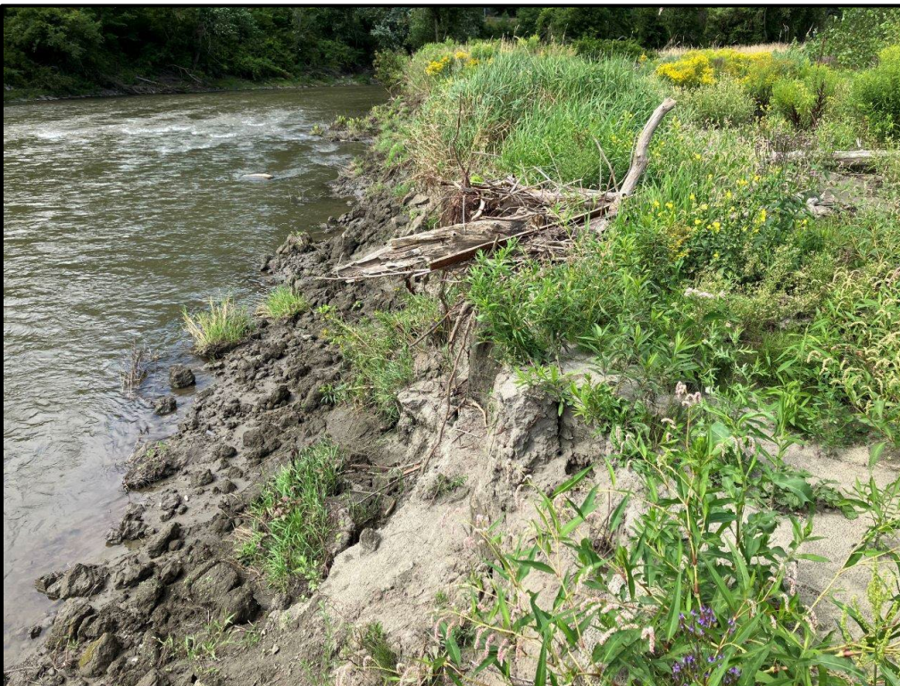
Plate 6. Close-Up of Low, Actively Eroding Riverbank, View North-Northwest
