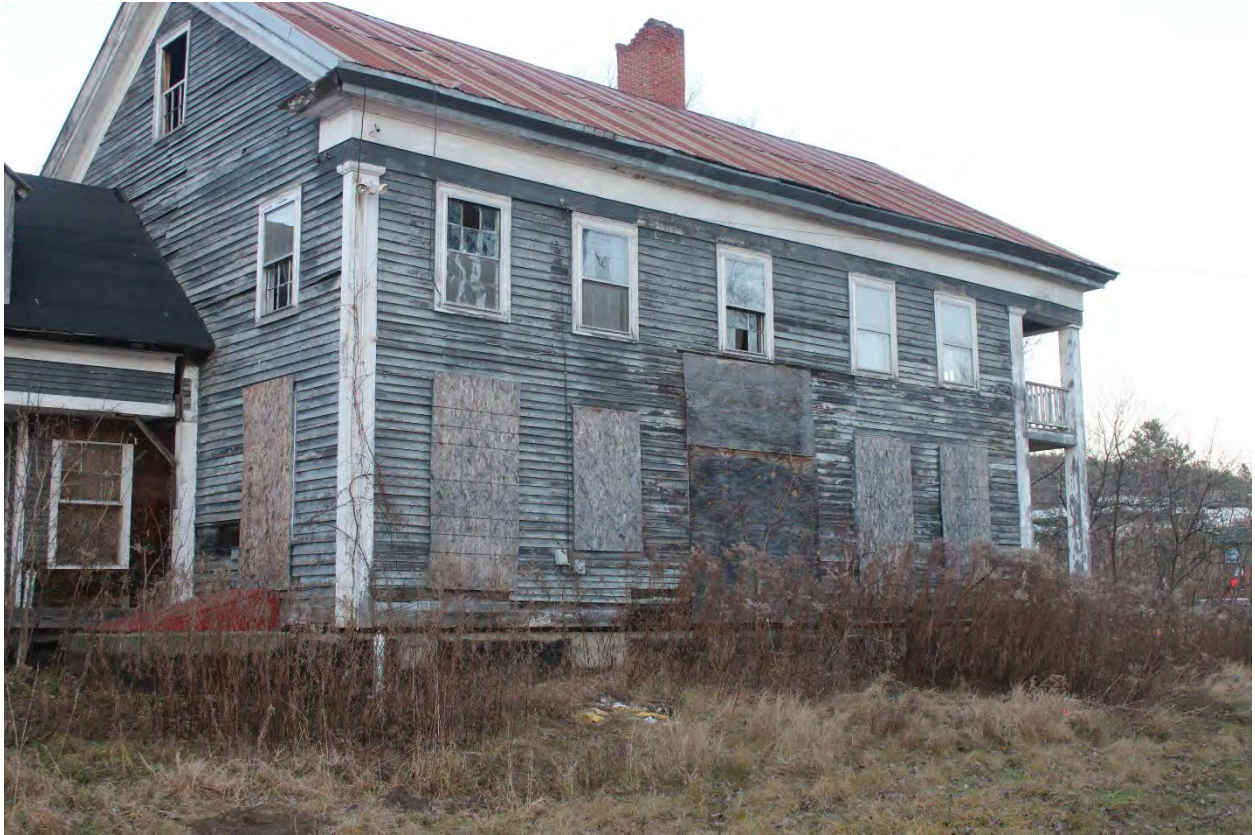
Figure 4. View approximately north of the Jacob Davis Homestead within the Jacob Davis House Demolition/Winooski Floodplain Restoration Project, Montpelier, Washington County, Vermont. Note the dilapidated nature of the structure, including the boarded windows, the missing chimney brick, and overall poor condition.
