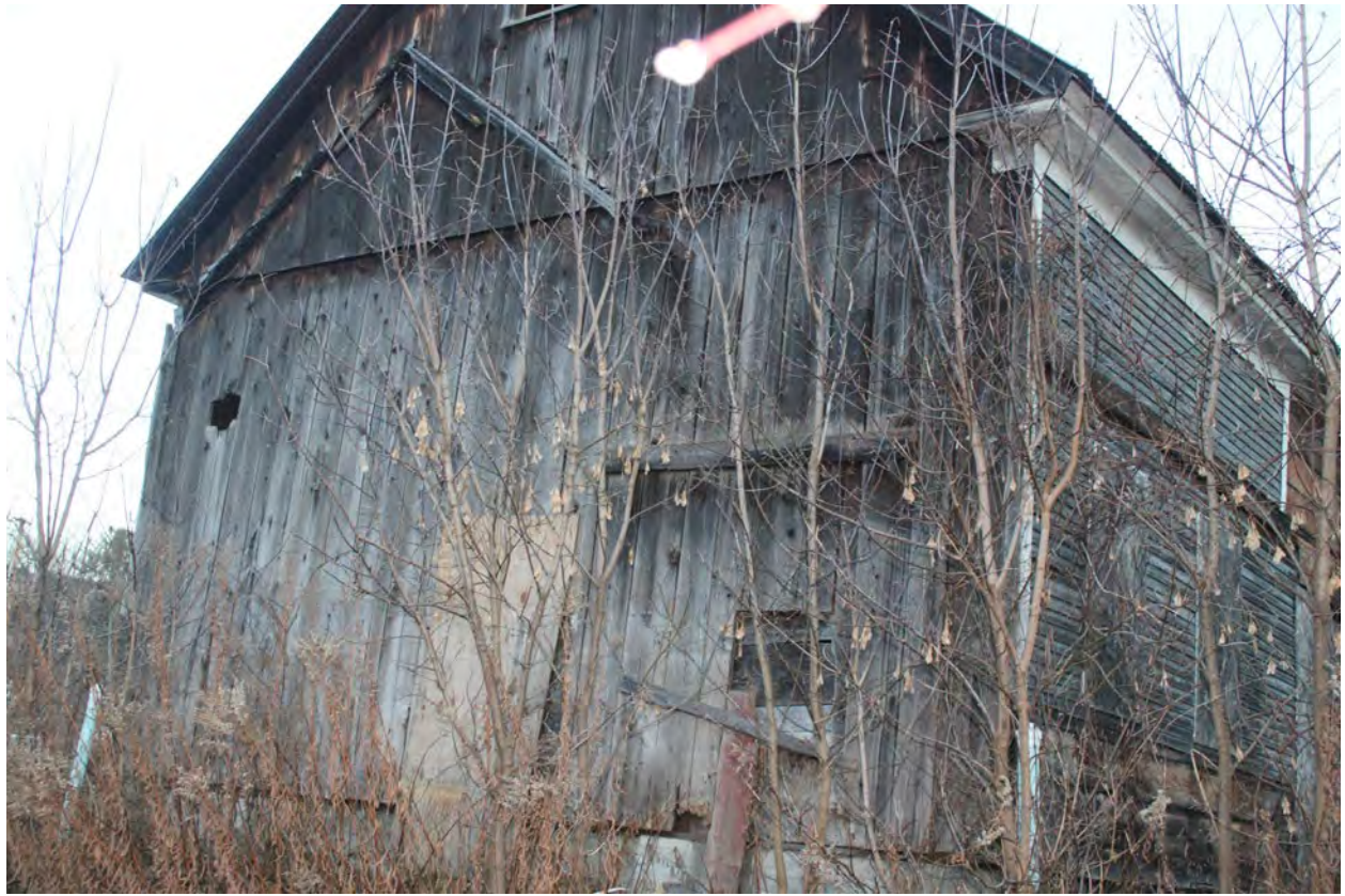
Figure 5. View east of the rear gable of the attached horse barn at the Jacob Davis House Demolition/Winooski Floodplain Restoration Project, Montpelier, Washington County, Vermont. Note the poor condition of the structure.
