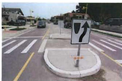
Median island/pedestrian refuge with cut-through but lacking detectable warnings
