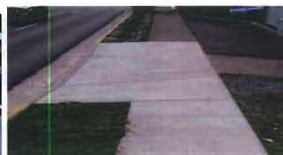
Driveway with steep cross-slope
