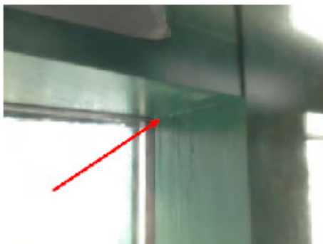
Photo No. 4 Test Specimen #2 Water Observed at the Corners of the Horizontal Mullions
