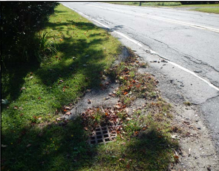
Photo 2. Catch basin that needs to be fitted with a riser.
