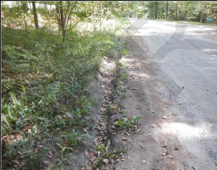
Photo 1. Roadside erosion in Hubbard Park
