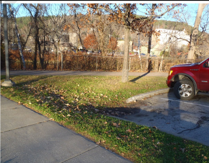
Photo 2: Sediment accumulation notes at corner of parking lot
