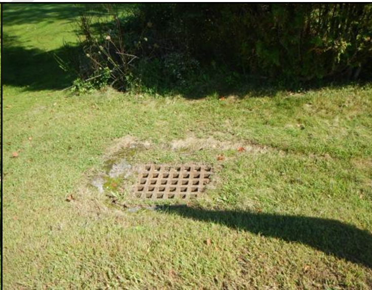
Photo 2. Erosion around catch basin.
