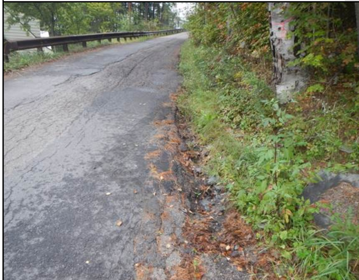
Photo 1. Erosion on roadside requiring ditch maintenance
