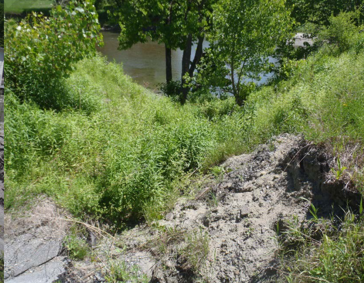
Photo 2. Visible evidence of active erosion.
