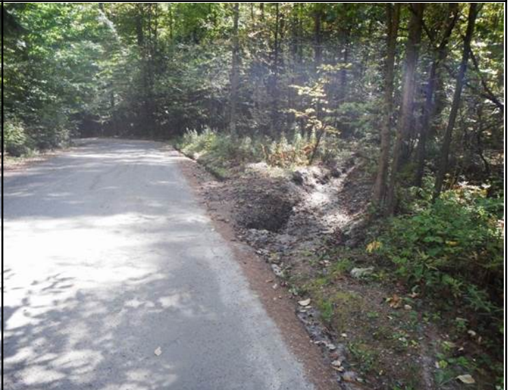
Photo 2. Roadside erosion in Hubbard Park
