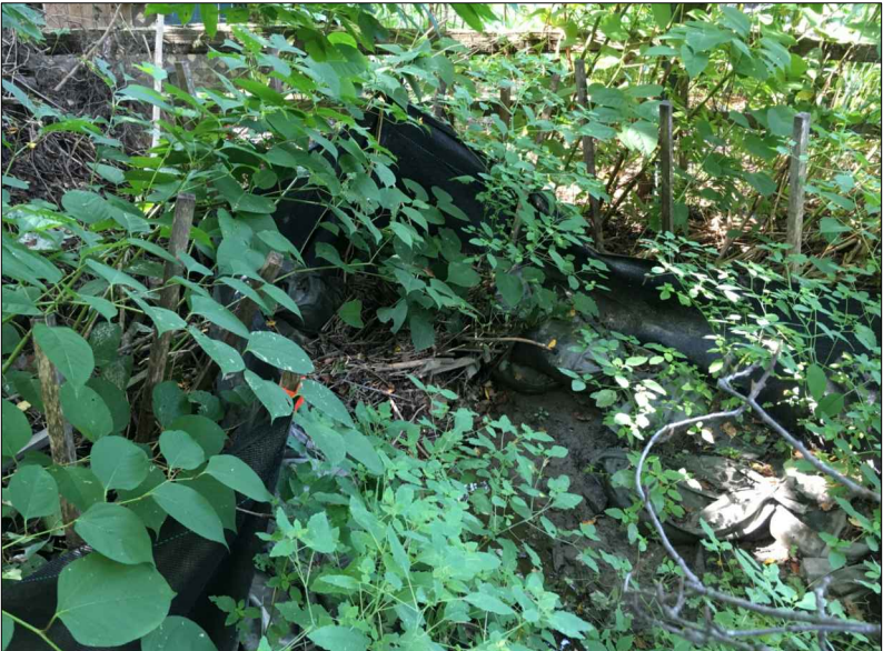
HA-08: UNKNOWN COLLECTION / OUTLET STRUCTURE IN SWALE
