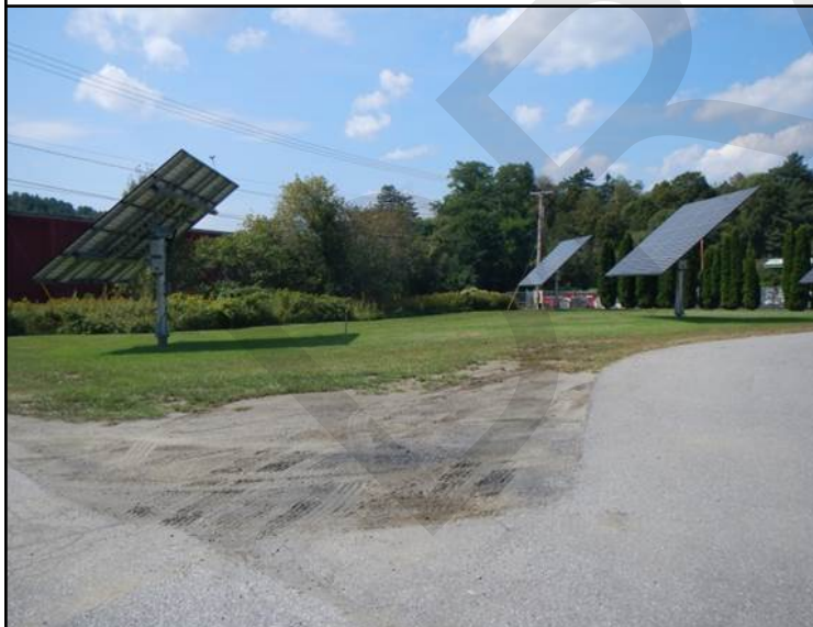
Photo 1. Solar panel installation that could be modified to incorporate stormwater management
