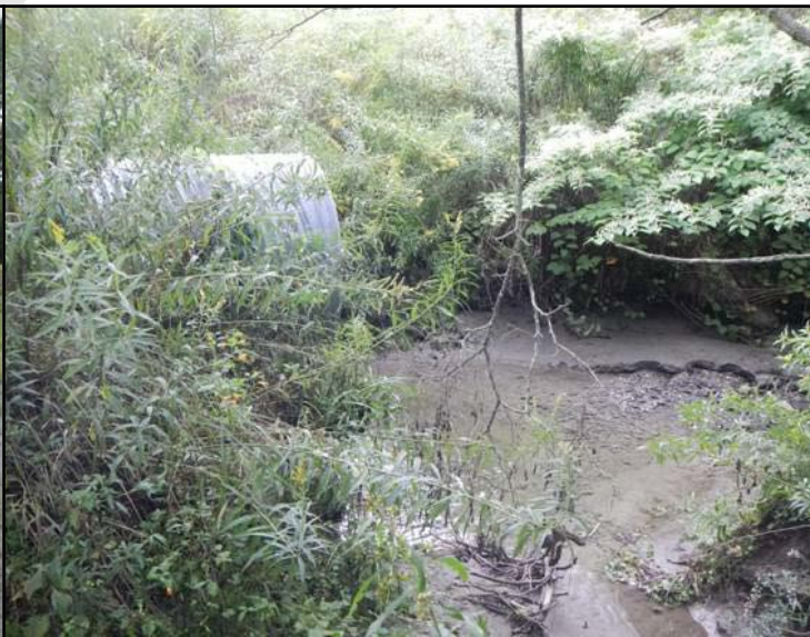
Photo 2. Culvert outlet pool. Note eroded banks.
