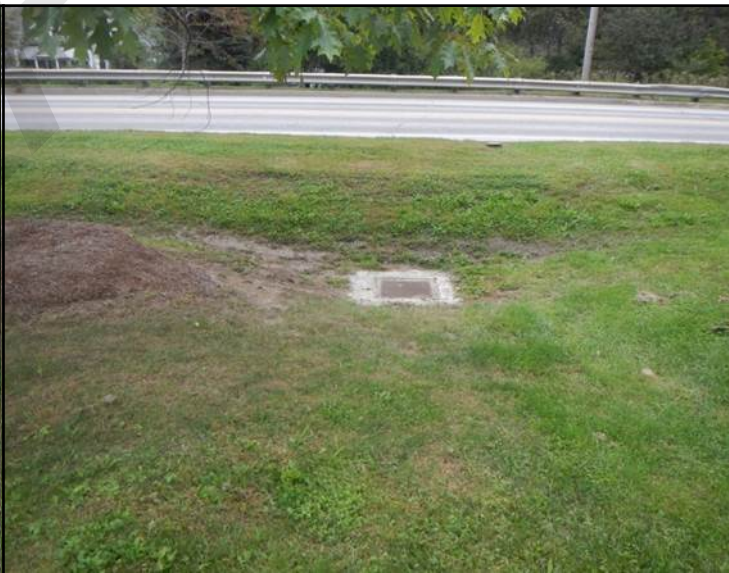
Photo 2. Catch basin that needs to be raised
