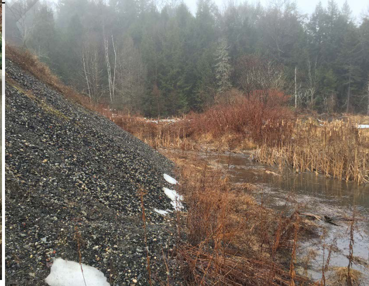
Photo 2. Material stockpile slumping into watercourse.
