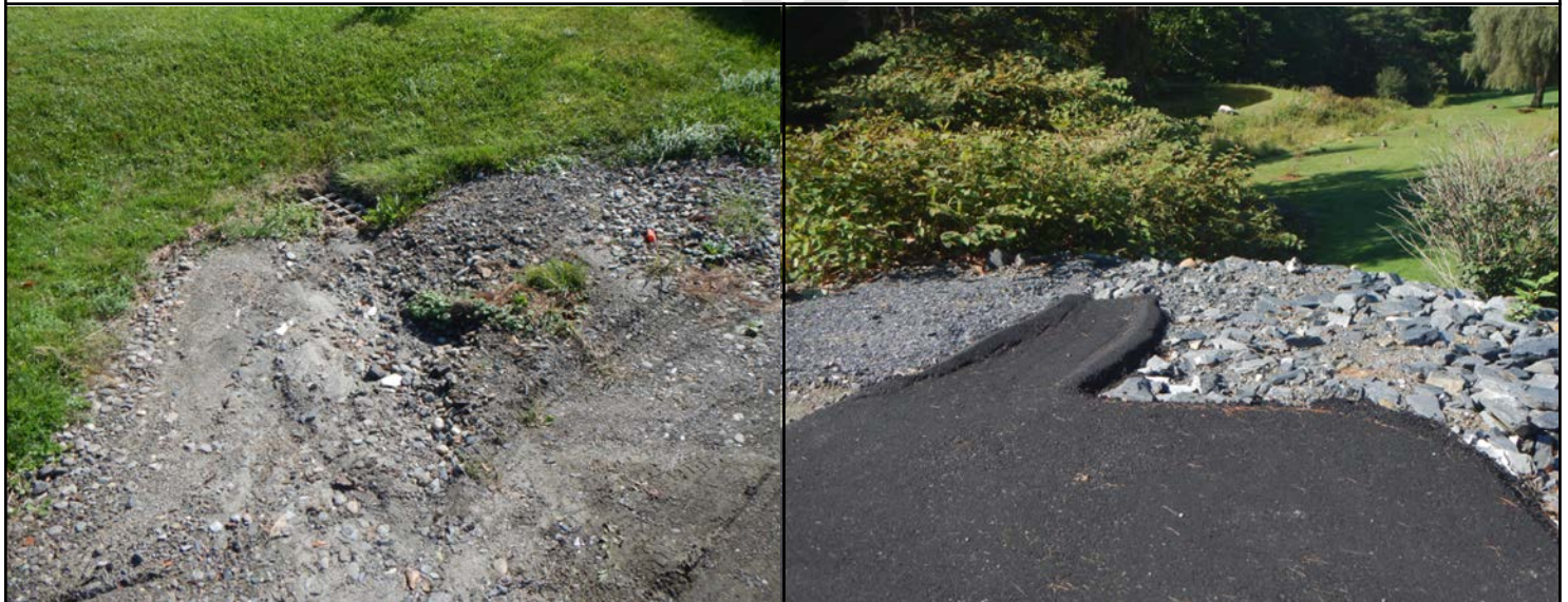
Photo 1. Erosion at catch basin
