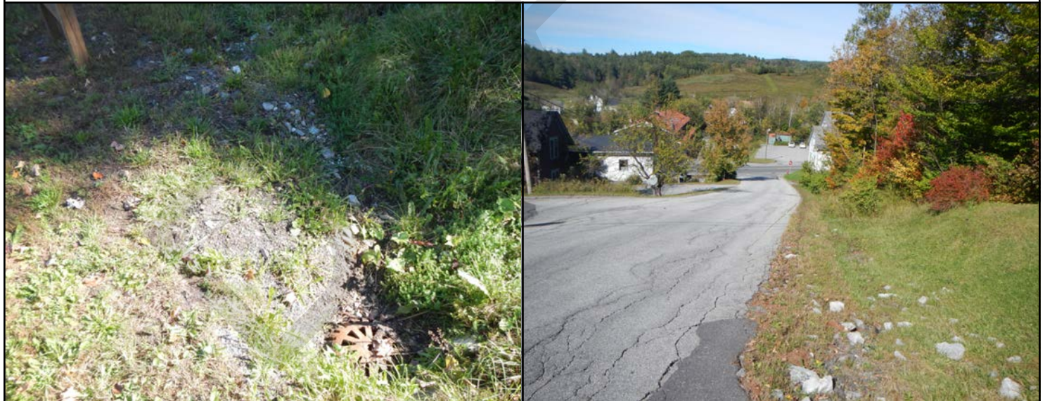
Photo 1. Catch basin and ditch could be improved.
