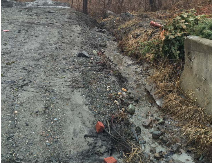
Photo 1. Erosion along haul road shoulder.
