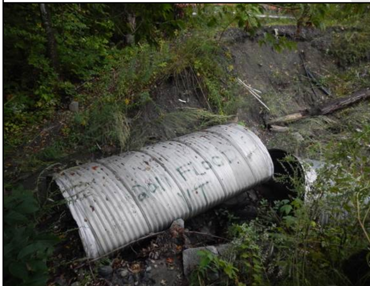
Photo 1. Damaged culvert and severe storm damage.
