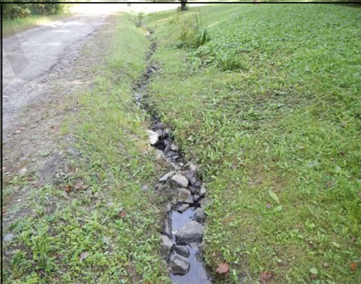
Photo 2. Ditch in need of repair.
