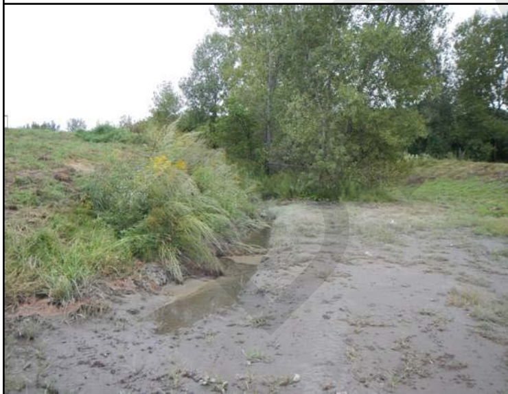
Photo 1. Shallow ditch and wet area reaching from the auto body service center parking lot to the culvert outlet pool
