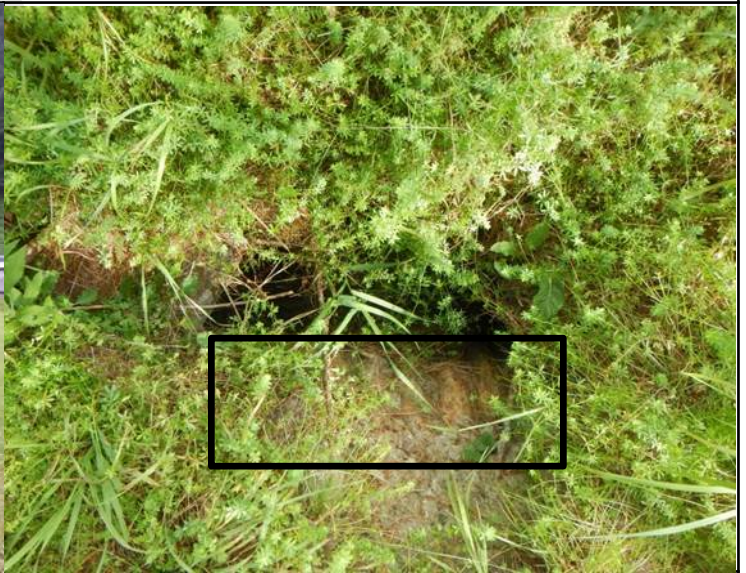
Photo 2. Exposed pipe (in box) and eroded area
