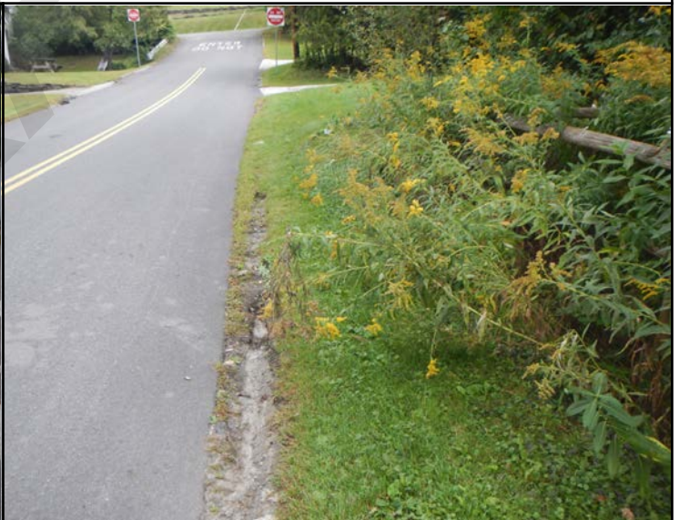
Photo 2. Minor erosion along Woodrow Ave.
