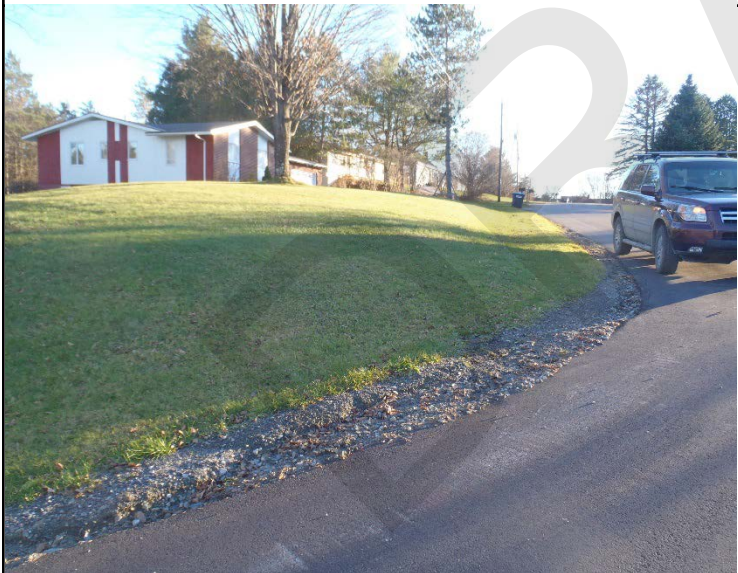
Photo 1. Erosion along the road shoulder
