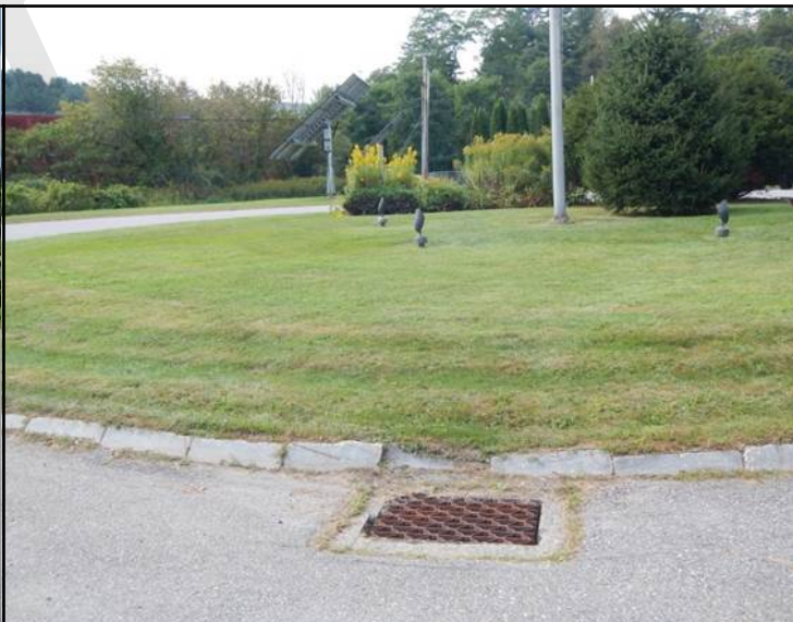
Photo 2. Catch basin that could be plated over (1 of 2)
