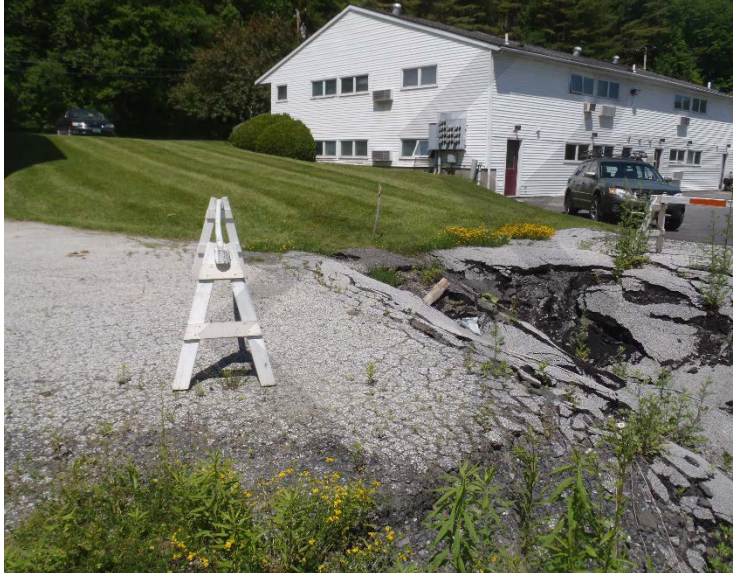
Photo 1. Damaged area where culvert used to be.
