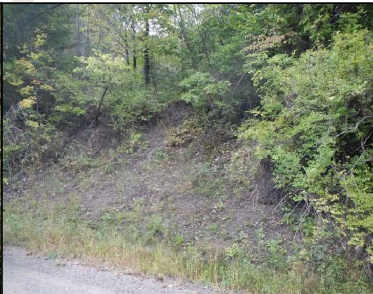
Photo 2. Erosion of area draining into the ditch on side of the road.
