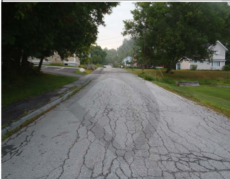
Photo 1. Harrison Ave is narrow with sidewalk immediately adjacent to the roadway.
