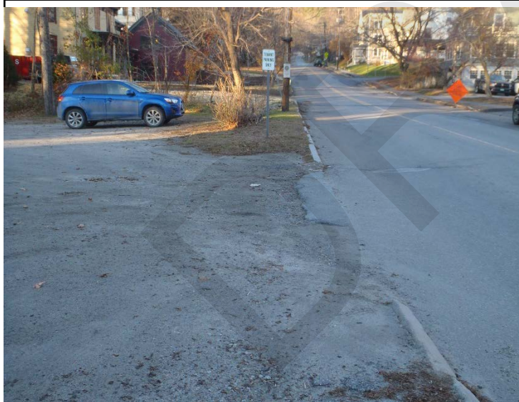
Photo 1. Runoff along the shoulder of Bailey Ave is accessing and eroding an off-street parking area.
