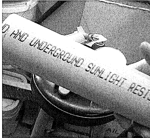
2-inch PVC tubing to protect extension chords
